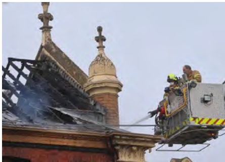
The building's roof was badly damaged.
