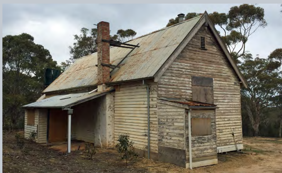
Disused Steiglitz State School No.1487 in poor state of repair, 2016. Photo: F. Gray
