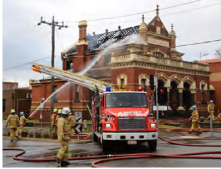
Fire has destroyed the roof of the building.
