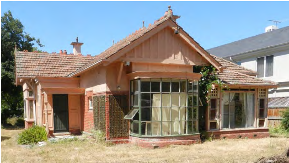
Above: 'Ngara' in 2015. There are signs that it has been broken into and vandalised. It is in danger of becoming yet another example of demolition by neglect. See back cover for exterior in 2013.
